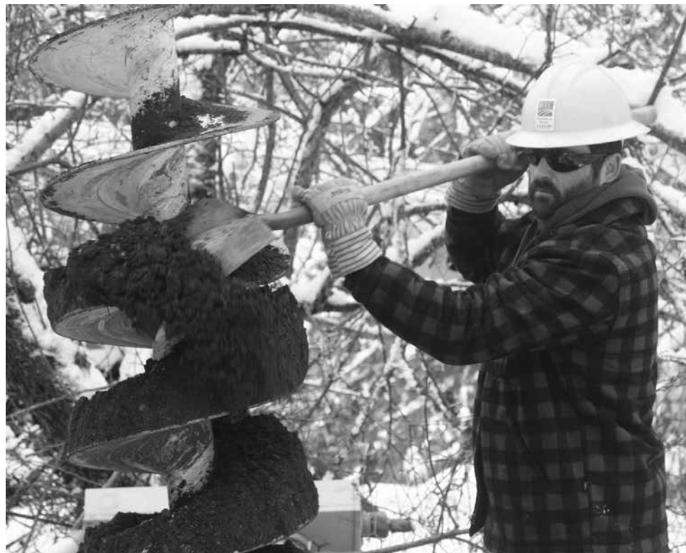
Line Worker Doug deGroseilliers pushes dirt from the blades of an augur that’s being used to carve out a hole for a replacement pole. The crew hit ledge a few feet down, but since options weren’t available for placing the pole it called for extra stabilization methods.
