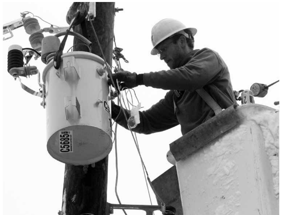
Setting a replacement pole is just the beginning of what must be done. Above, Line Worker Hans Pope-Howe attaches the transformer that will reduce the power voltage for this member. Further tasks included attaching the transformer to the underground service to the house, and securing hardware to the pole. Such extensive work was needed in places all over WEC’s service territory.
