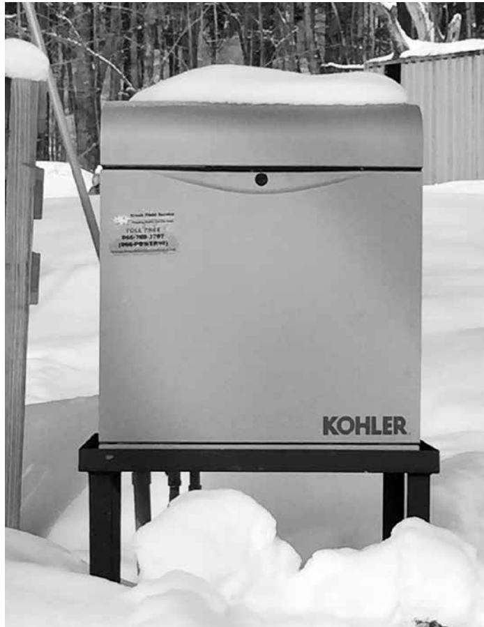
A Kohler generator installation is ready for any weather. Brook Field Systems owner Jim Brochhausen said the permanent, automatic, propane-fueled generators he sells perform flawlessly.
