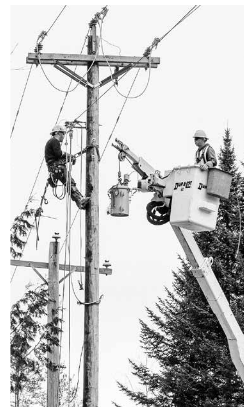
'I have hold of this if you would like to...' WEC lineworkers hover over Willey Hill Road after elevating power lines.
