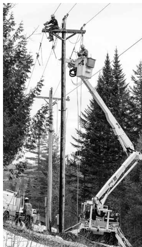
Specialized equipment supports WEC line crews when and where possible. Remote placements and stormy conditions pose a greater challenge.
