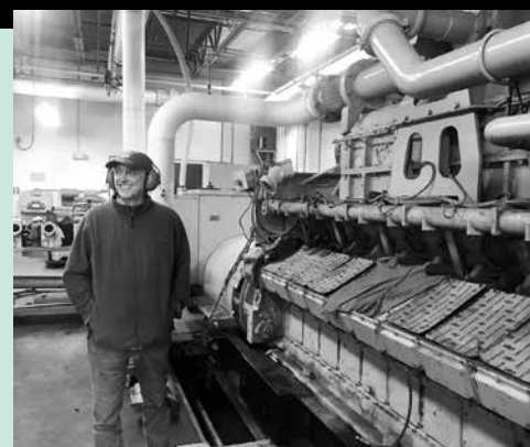
WEC President Stephen Knowlton tours WEC's Coventry landfill gas generation plant during WEC's open house September 17.
