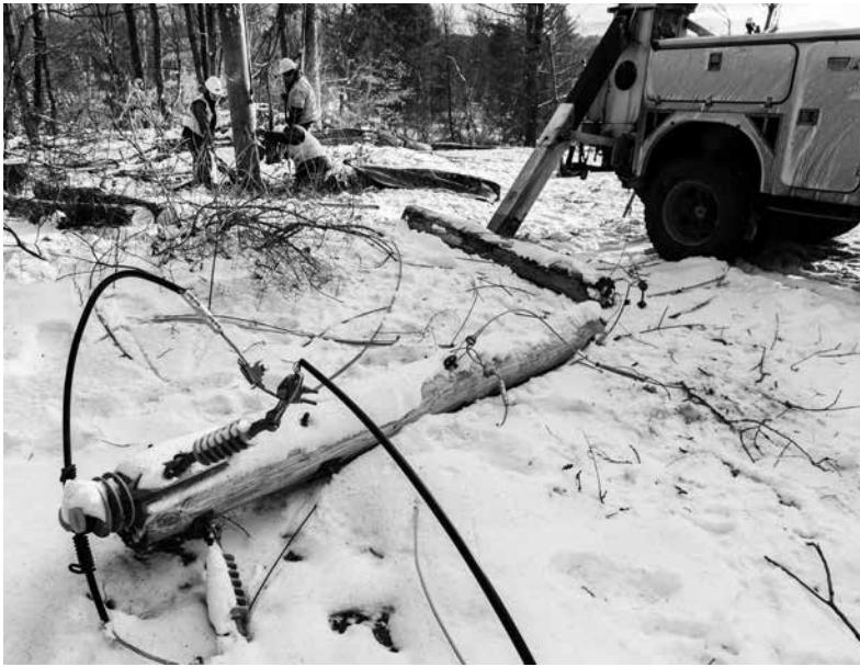
Left: Crew from Vance Line Construction of West Danville puts up a new pole off Cummings Road, East Montpelier.
