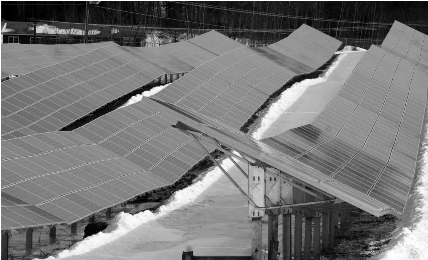
The solar panels roll and undulate across the contours of the land at the Williamstown Solar Farm.
