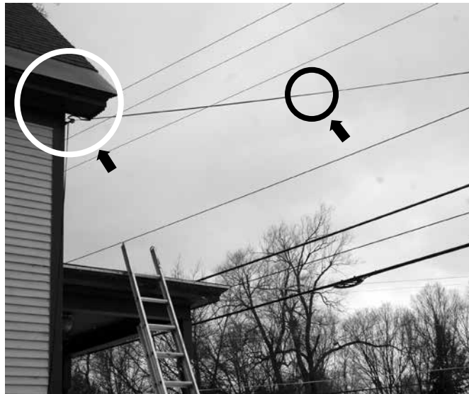
The owner of this home had recently shoveled 18 inches of snow off the porch roof shown here. Note the proximity of the aluminum extension ladder to the home's electric service entrance (circled), as well as other wires and cables. Homeowners need to be very mindful and cautious in circumstances like this.
